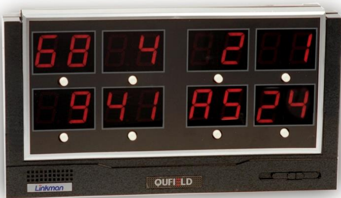
Display switchboard for the control room
